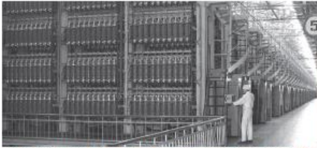
Interior view of a cascade hall of Russia's Novouralsk centrifuge enrichment plant. The facility has a capacity of more than 10 million separative work units per year.
