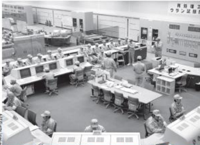
Control room of Japan’s spent fuel reprocessing plant at Rokkasho, Dec. 21, 2004. The facility has a design throughput of 8,000 kilograms of plutonium per year.
